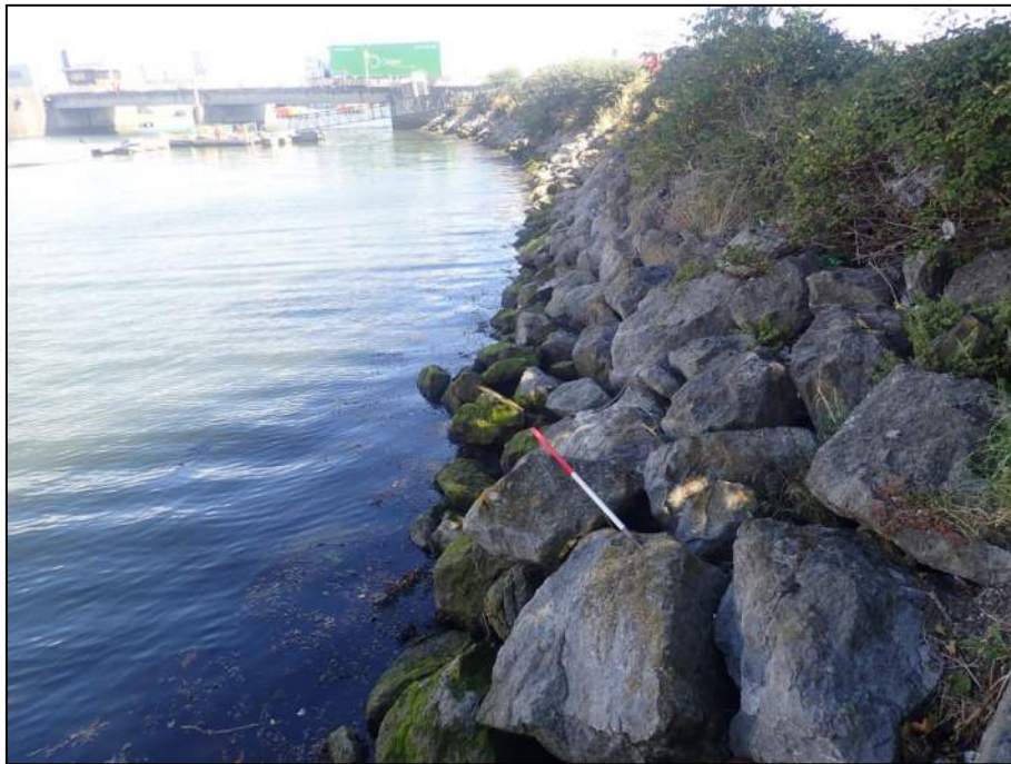
Plate 21: East-facing view along rock-armour that delineates the southern shoreline on the upstream side of Tom Clarke Bridge (1m scale).
