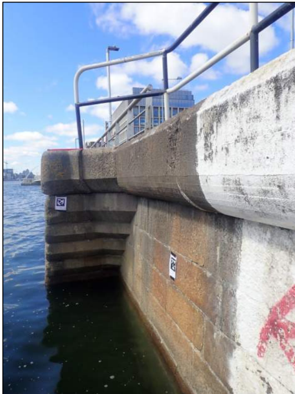
Plate 18: West-facing view of bullnose terminus to cascading masonry on the upstream side of river access steps (RAS01).
