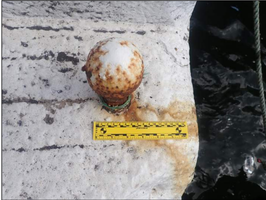
Plate 17: Detail shot showing example of boat tie-off fitting, inset into every second step (150mm scale).
