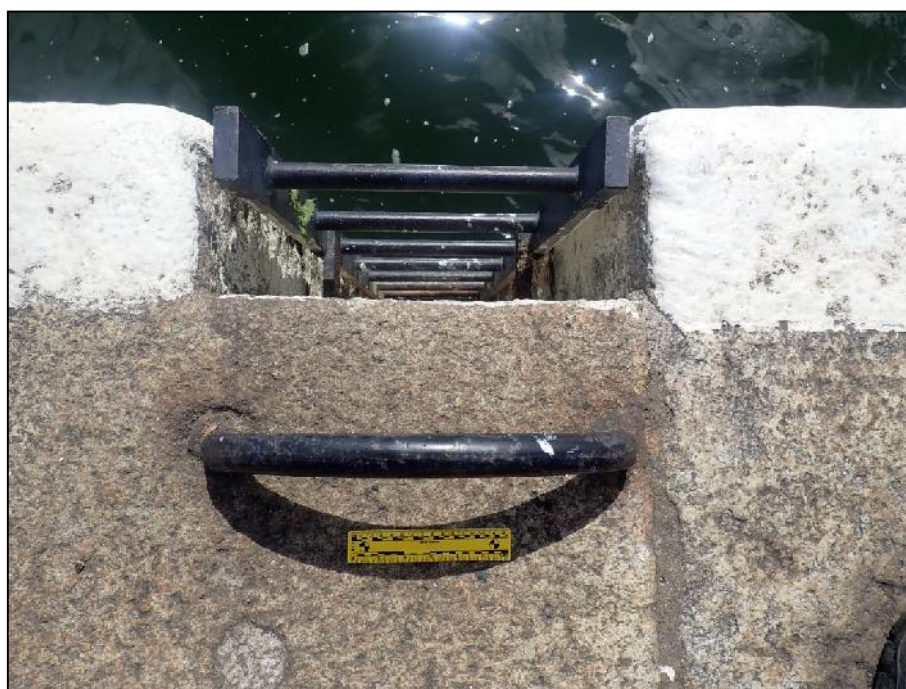
Plate 12: Recessed river access ladder (AL01), located at ITM 717965E, 734391N (150mm scale).
