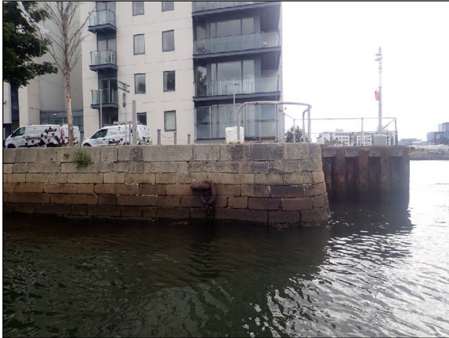
Plate 23: South-facing view of masonry quay wall and associated mooring ring, located at ITM 717924E, 734211N.
