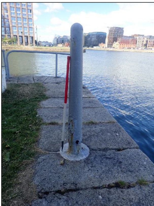
Plate 26: Partial remains of a derrick or similar lifting structure, inset into capstone area of quay wall (1m scale).
